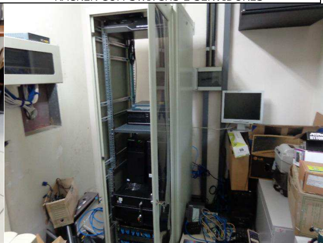
RACKER COM SWITCHS E SERVIDORES
